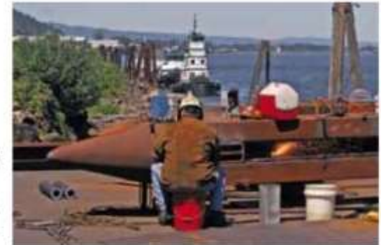
L.E. BASKOW / PORTLAND TRIBUNE Chris Johnson of Advanced American Construction Inc. welds and repairs spuds for use on a crane barge. About 40,000 people have jobs at the Portland Harbor, many of them in industrial occupations.
